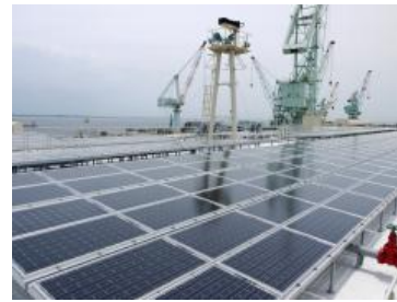
HIT solar modules covering the garage deck
