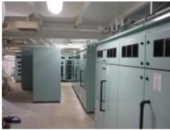
Battery room storing lithium-ion batteries
