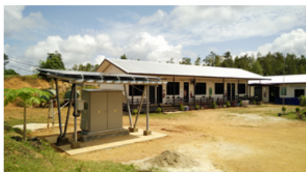
Power Supply Station installed in Indonesia as part of the project (West Kalimantan)
